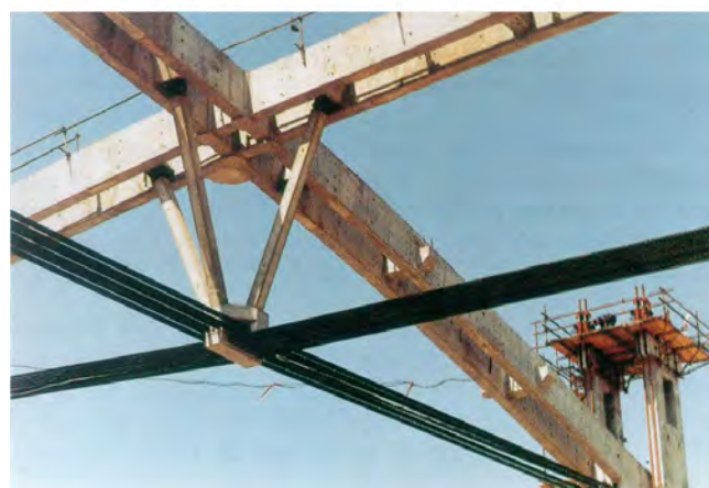
Figure 4. The roof structure of sports hall Belgrade Arena (1992) – two-chord externally prestressed reinforced concrete girders, spans 132.7 and 102.7 m, covering the area of 15000 square meters
