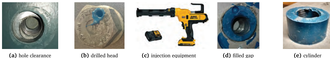
Figure 4. Installation process of injected bolts from the hole clearance to the disassembling
