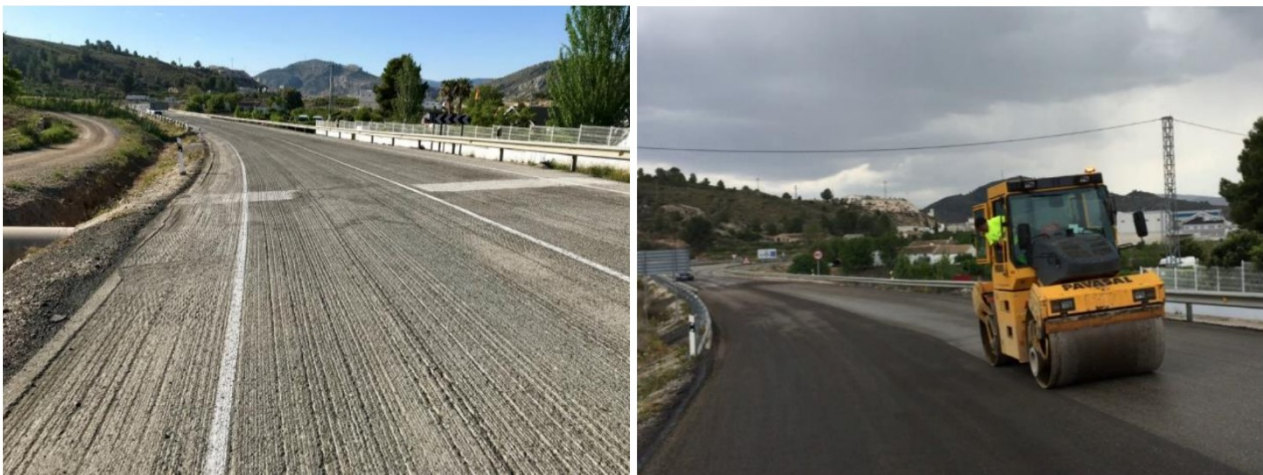
Figure 7. On the left, milled surface before laying binder layer; on the right compacting the binder layer
