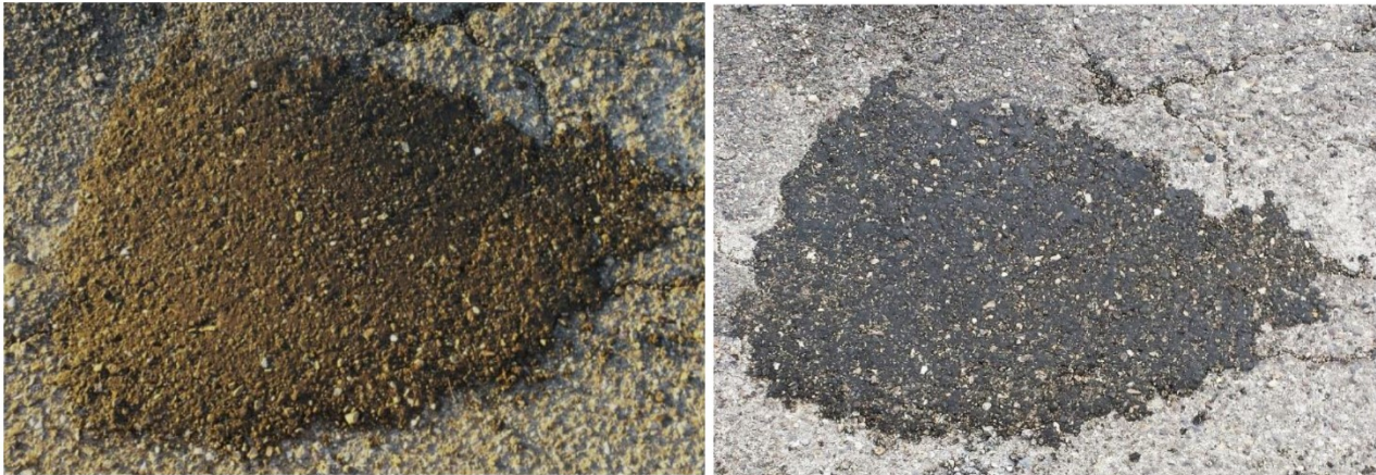
Figure 6. On the left, placing the mixture for patching a pothole, first day. On the right compacted surface after 14 days
