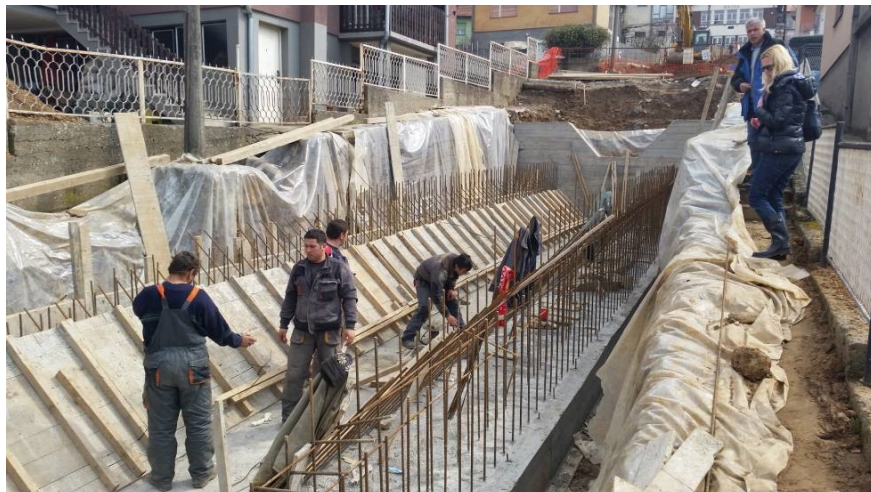
Slika 6. Izgradnja glavnog kanala kroz stepenice u Tekiji, mart 2015. Figure 6. Construction of the main flood channel in Tekija, March 2015
