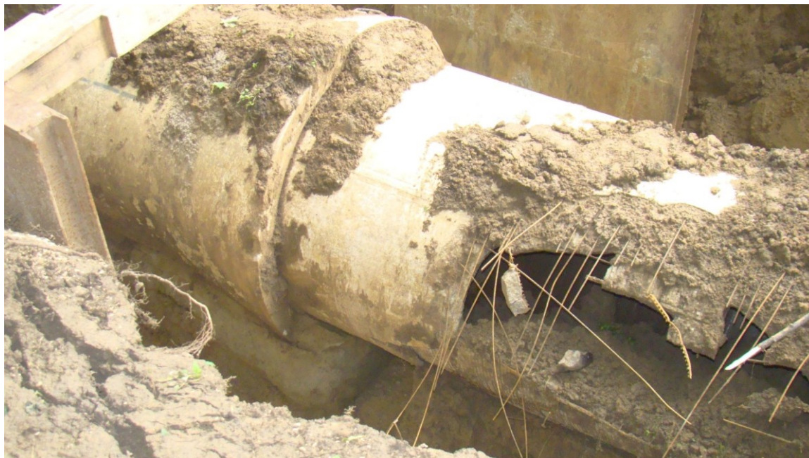
Slika 11. Mesto havarije cevodova AB1200 u blizini rezervoara “Petlovo brdo”. Figure 11. Ruptured reinforced pipe DN 1200, near the “Petlovo brdo” reservoir.
