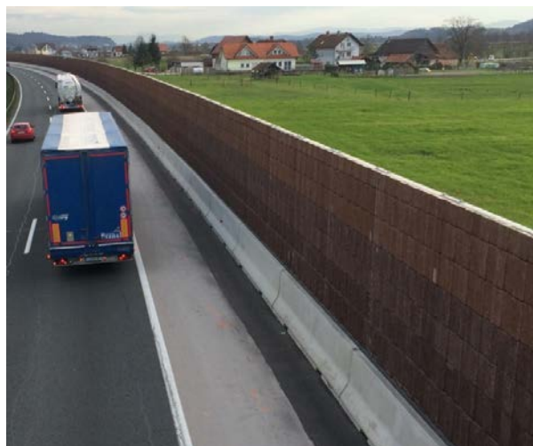
Figure 3. Free-standing noise barrier in Vrhnika, Slovenia Source: Photograph © DELTA BLOC International GmbH
