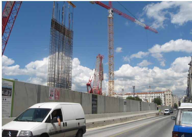
Figure 13. Temporary application of DB 80 LSW-R, Italy Source: Photograph © DELTA BLOC International GmbH
