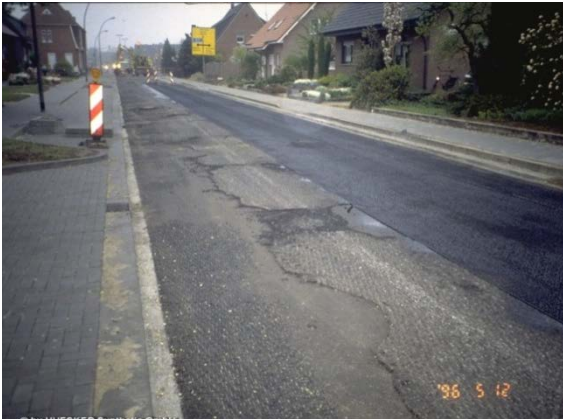
Figure 4. Condition after milling in May 1996
