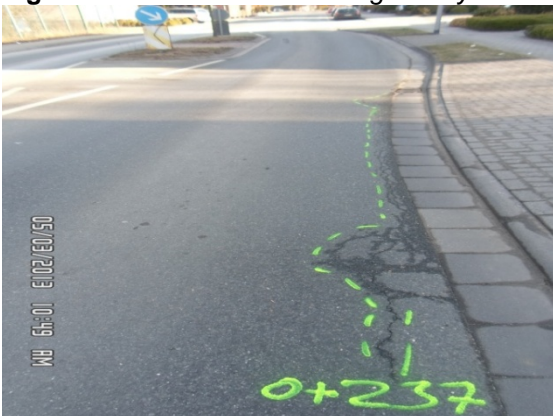
Figure 6. Cracking resulting from road works
