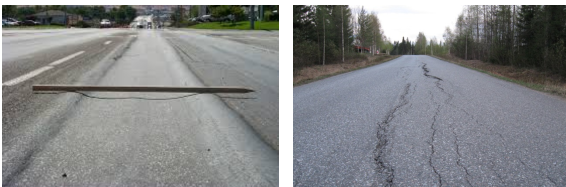
Figure 6. Rutting deformation and fatigue cracks
