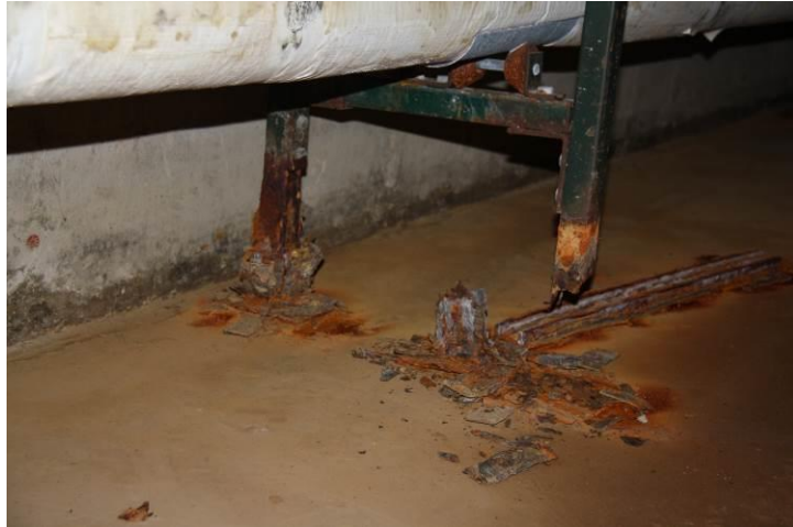
Figure 5 - Deterioration observed at steel pipe rack bases
