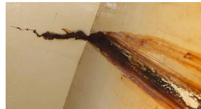
Figure 13 – Slab POS 5; crack above expansion joints, traces of dark liquid leakage
