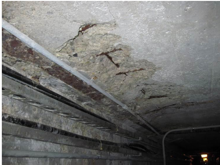
Figure 4 - Deterioration observed on the underside of the roof slab
