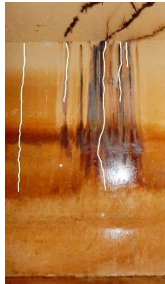
Figure 8 – Series of vertical cracks, linked with cracks in the upper slab
