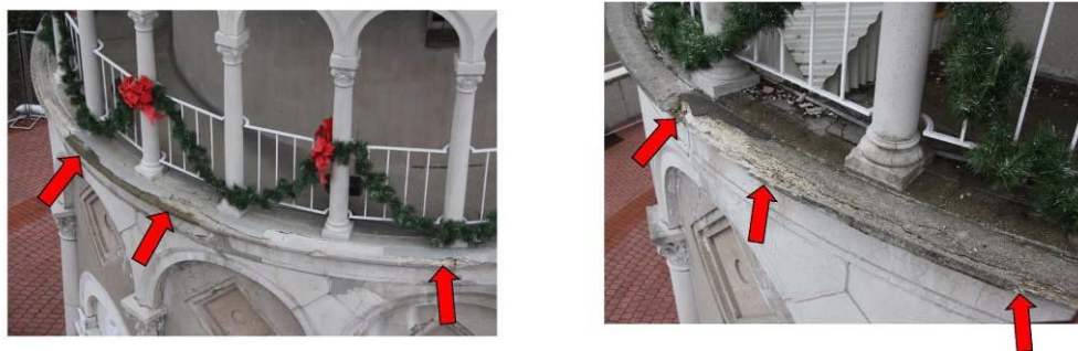
Figure 5 - Distressed precast coping at the 2nd floor
