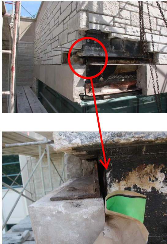
Figure 8 - Overall and close up view of detached shelf angle from structural beam and cracked limestone panel at the back side due to corrosion of shelf angle
