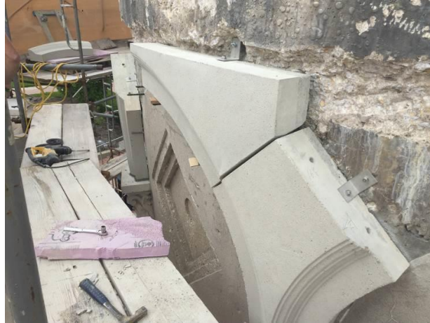
Figure 7b - Close up view of the new precast arch panels during the installation
