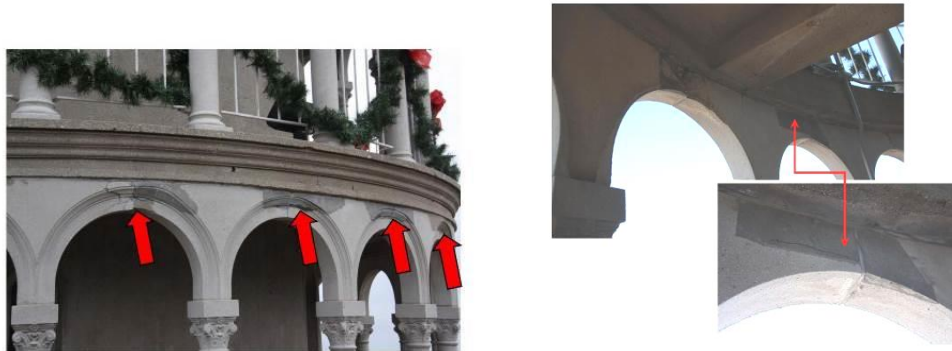
Figure 6 - Typical distress observed at precast concrete arch panels at typical floors
