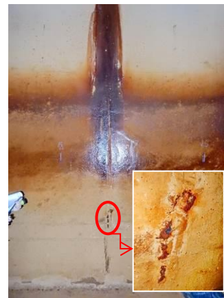
Figure 10 – Appearance of damaged expansion joint, inner side of wall
