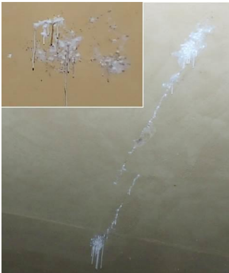
Figure 12 – Slab POS 12, cracks parallel to main axis, leakage of \text{Ca}(\text{OH})_2 , white stalactites
