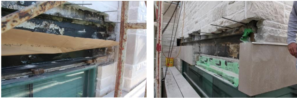
Figure 12 - Repair 6, repairing of steel shelf angles / window lintels at building built in 1953.
