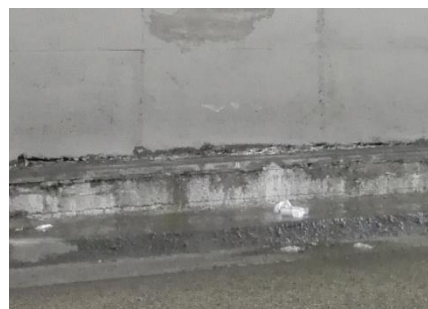
Figure 5 - Water ingress at a joint of concrete building.
