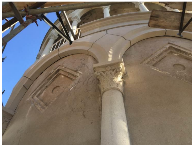
Figure 7c - Close up view of the installed new precast arch panels column capital, and coping above it
