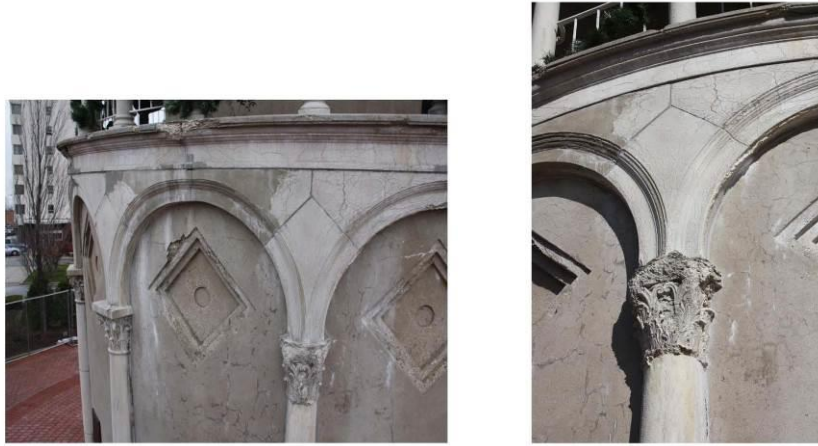
Figure 4 - Extensive Freeze thaw damage observed at precast concrete arches
