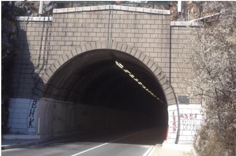
Figure 1 - The “Budosh” tunnel before repair.
