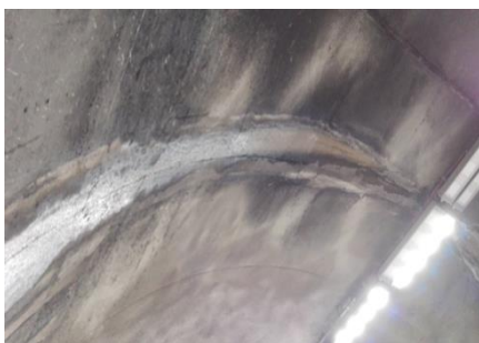
Figure 4 - Water ingress at the crown
