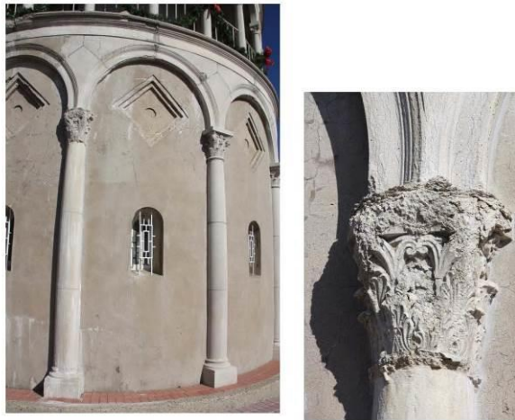
Figure 3 - Freeze thaw damage observed at precast concrete column capital
