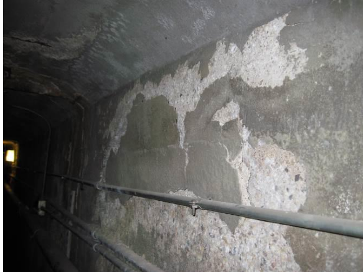
Figure 3 - Deterioration observed on concrete walls
