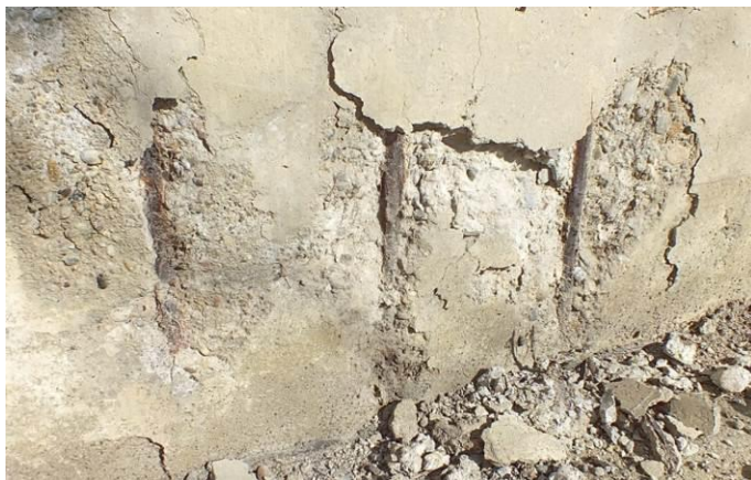
Figure 9 – Insufficient thickness of the concrete cover, cracking, delamination and falling of the concrete, reinforcement corrosion in the lower part of the wall
