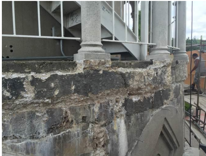
Figure 7a - Close up view of removed precast arch panels at the 2nd floor
