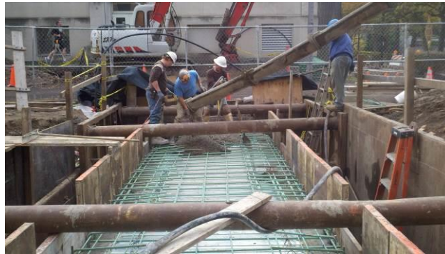
Figure 9 - Repair Option 2, partial replacement of tunnel structure. Installation of new roof slab
