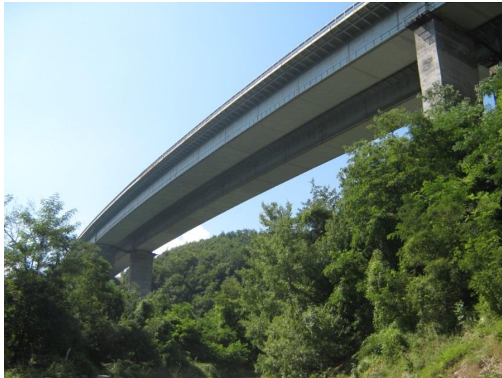
Fig.5 Viaduct 2 “Hemus” highway, 27.500km. (Courtesy of prof. M. Minev and prof. P. Staykov. With permission.)
