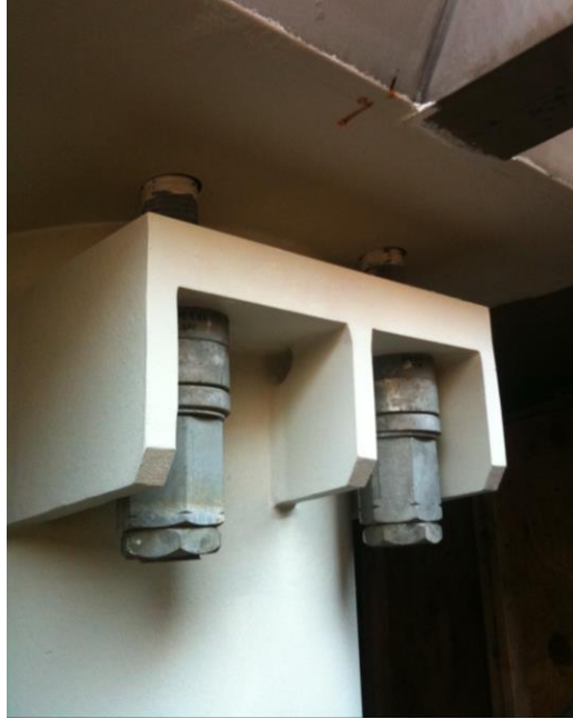
Figure 21. Weld 6.2 retrofit bracket
