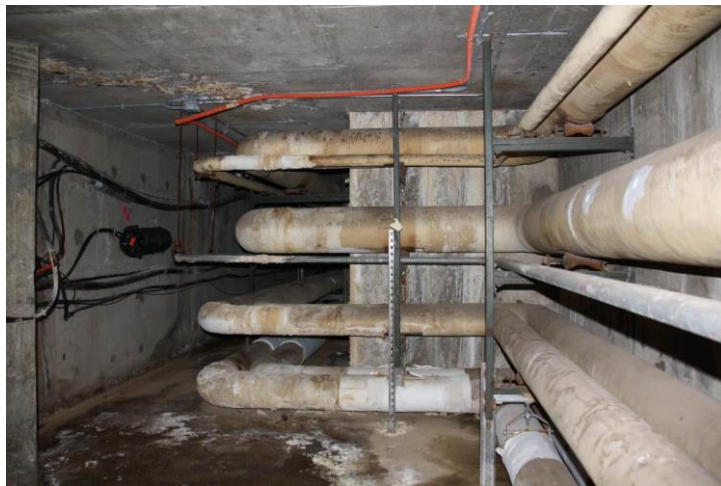
Figure 6 - Actively leaking crack in the roof slab and water ponding on the floor
