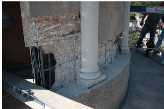
Figure 11 - Partial and full depth wall repairs of concrete core at 8th floor
