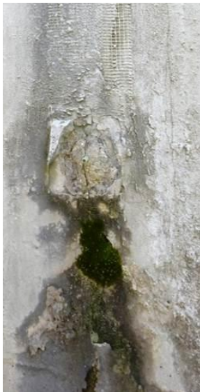
Figure 7 – Vertical crack, leakage, moss, previous repair - T2
