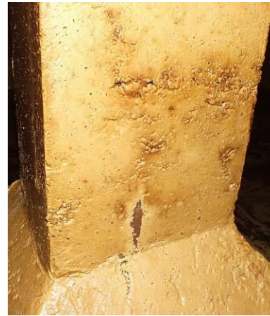
Figure 16 - RC column, local peeling of the protective coating
