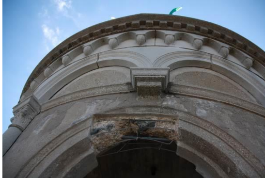
Figure 10 - Repair of delaminated cast in place concrete arch on the 8th floor
