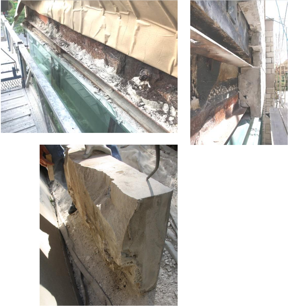
Figure 7 - Severely corroded steel shelf angle and cracked and spaled limestone block due to corrosion
