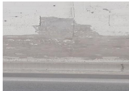
Figure 3 - Damages to the protective coating of the concrete surface
