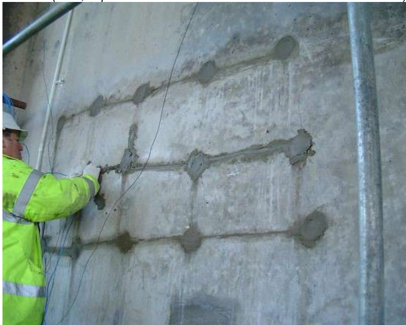
Slika 9 - Izgled zida posle ugradnje distribuiranih diskretnih anoda Source: (Izvor, The Principles and Practice of Galvanic Cathodic Protection for Reinforced Concrete Structures Technical Note 6 , G Sergi, J Broomfield and N Davison)
