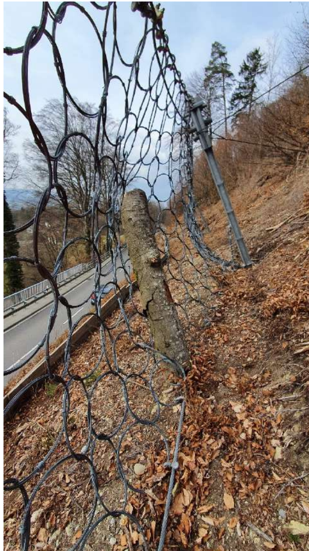
Figure 10. Cutting of a tree trunk after clearing and grubbing of vegetation around the construction. Source: (Gebrugg AG)
