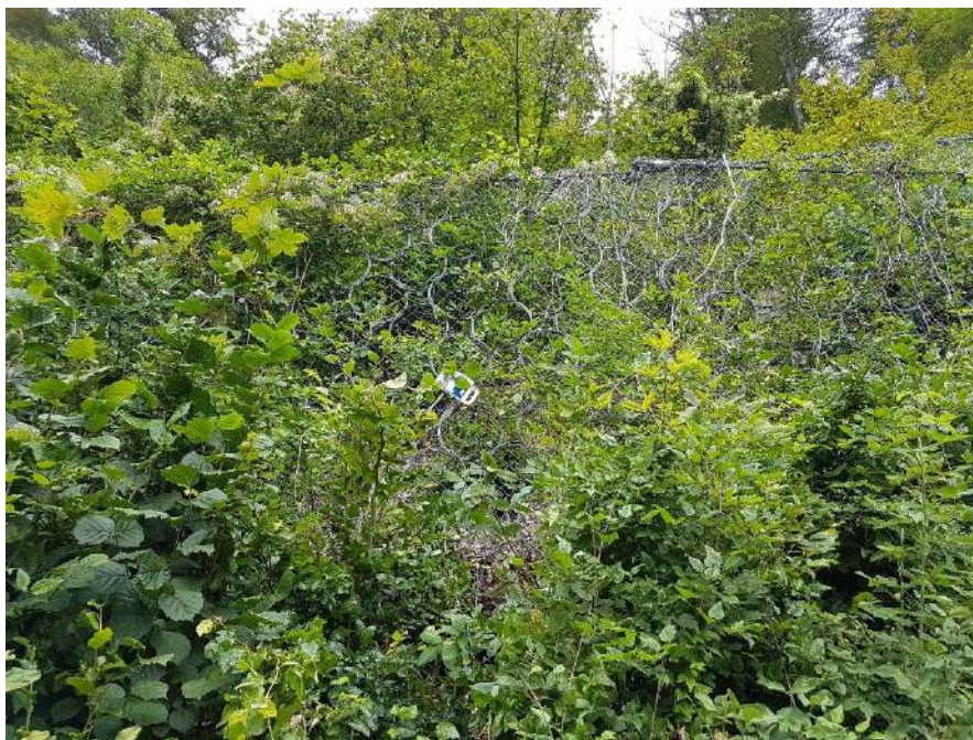
Figure 6. Rockfall protection barrier disappearing into the vegetation Source: (Geobrugg AG)
