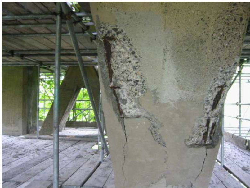
Slika 4. Primer „prstenaste“ anode – korozijska se nastavlja oko popravke betona; Source: (Izvor, The Principles and Practice of Galvanic Cathodic Protection for Reinforced Concrete Structures Technical Note 6, G Sergi, J Broomfield and N Davison)
