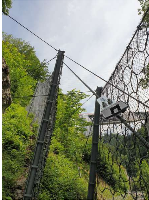
Figure 5. Guard mounted on the support cable of a rock-fall protection structure. Source: (Geobrugg AG)
