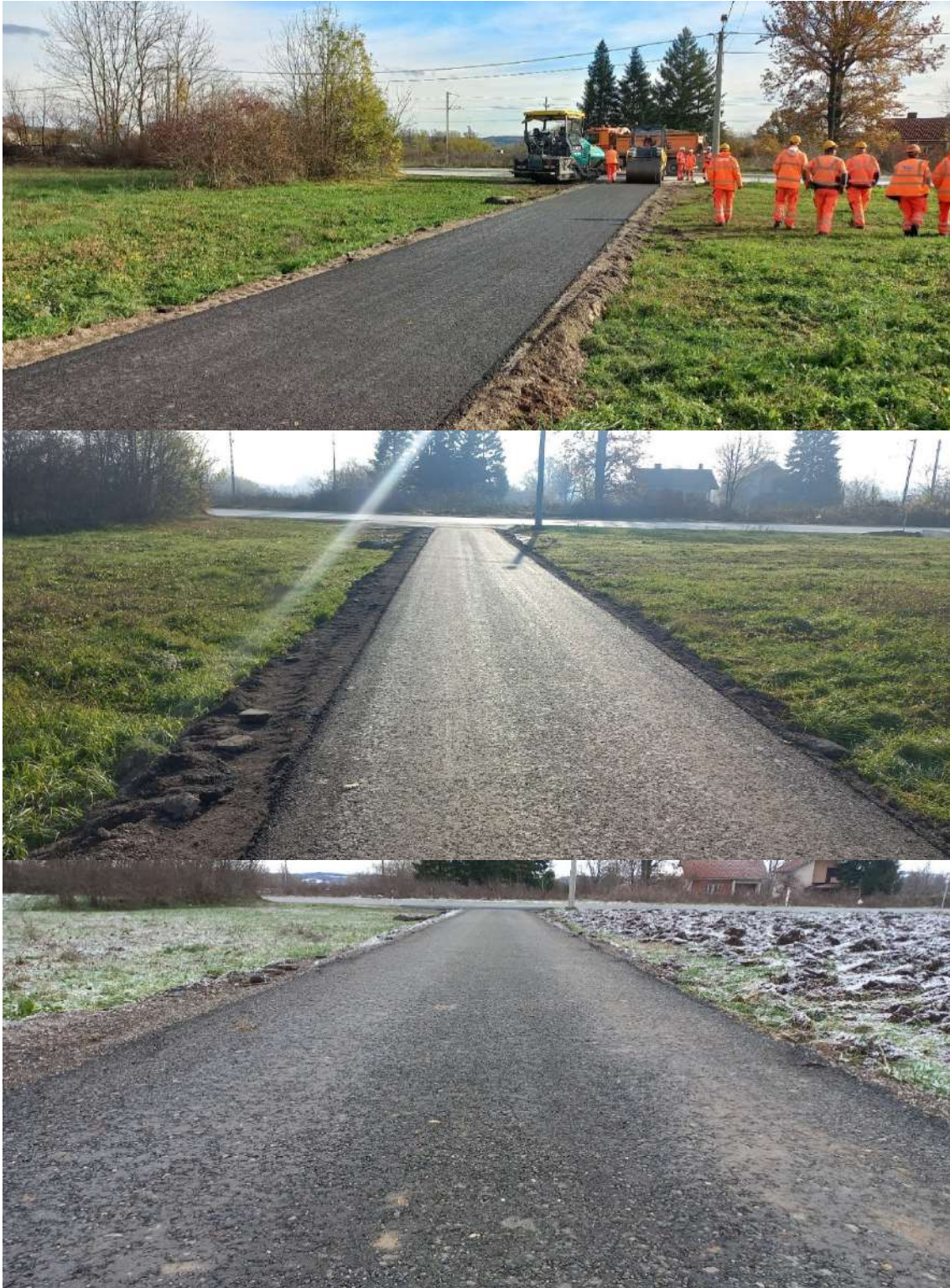
Figure 6. The test track during time. From the top: execution day, after 7 days, after 2 months
