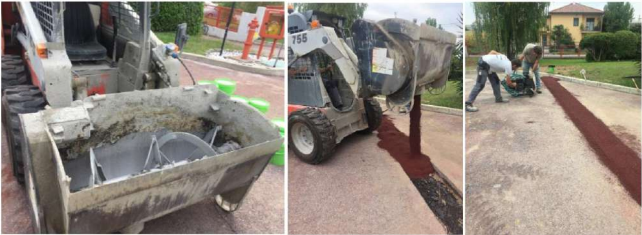
Figure 10. From right to left mobile mixer and bucket for hauling mixtures, placing the mixture into the cut, cleaned and prime coat covered repair zone, and final patched zone after compaction
